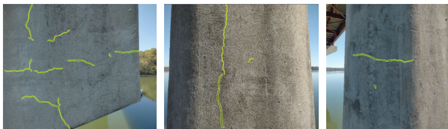
Fig. 3: Images of Pier 5 were captured using the UAS and subsequently annotated to highlight surface defects
