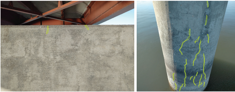
Fig. 4: Enhanced UAS-captured images of Pier 30
