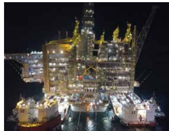
Fig. 2: The Hebron float-over and topsides-GBS mating operation. The project set an industry record for the heaviest marine float-over and topsides-GBS mating operation 3
